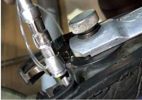
Fig. 4. Injection connectors are installed at each cable end to create a fluid access point for injecting silicone gel into the cable's conductor.
