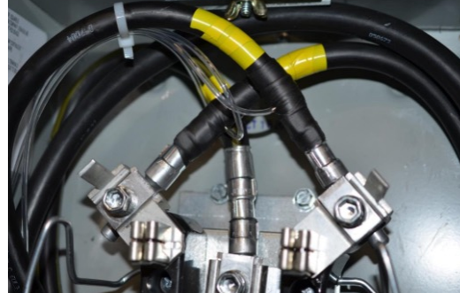
Fig. 5. Injection connectors installed in a residential 200A meterbox. Tubes are routed to the temporary collection tank.
