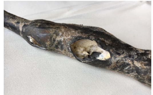
Fig. 1. Full loss of ampacity of a secondary service cable due to corrosion of the aluminum conductor.
