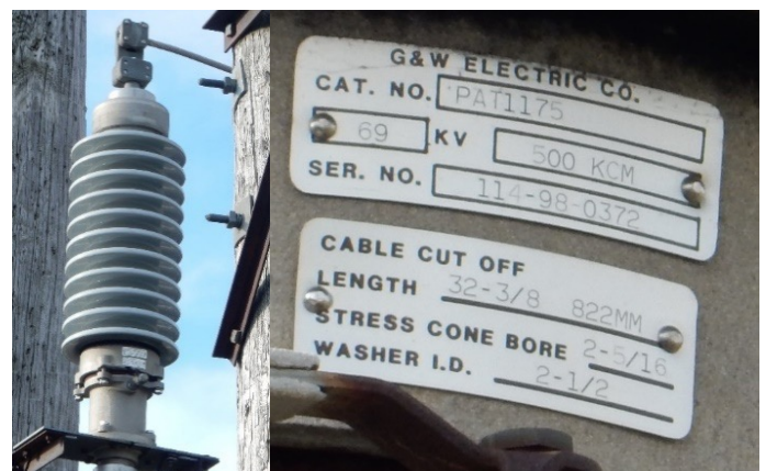
Figure 2: Photograph collected from aerial drone detailing the pole-top termination manufacturer's part numbers and specifications.
