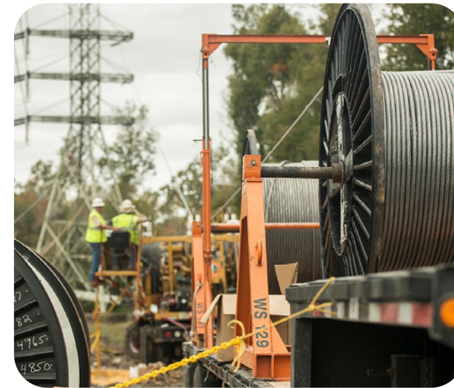
Figure 3: Pulling the conductor to ground to install the traveling ground is commonly done using a single rope. This could kink the conductor if tension was high enough. Use a 28x diameter guide roller, or slacken the conductor if it needs to be lowered to install the traveling ground. Photo courtesy of CenterPoint Energy.
