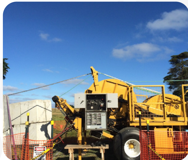
Figure 1: Example of a situation where bending is excessive even for ACSR. In this case, the payout reel is located downslope from the bull wheel, and the conductor bending angle is 35° around a four (4) inch roller. Photo courtesy of Trans Power New Zealand.
