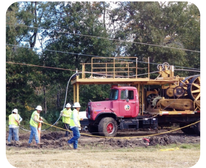
Figure 4: It is OK to drape slack conductor across a small roller. This would not be acceptable if the conductor was under tension or if the crew was pulling the tail to install a fitting.
