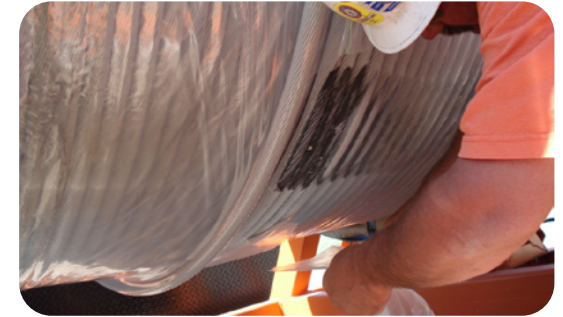
Figure 21: Water stain on conductor.
