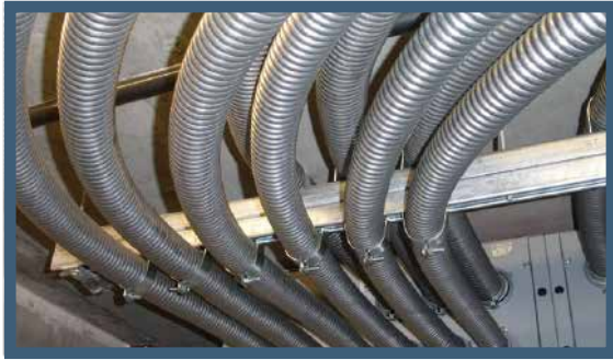
MC cable using strut support systems
