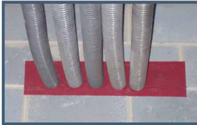
MC feeder cable in wall with fire stop
