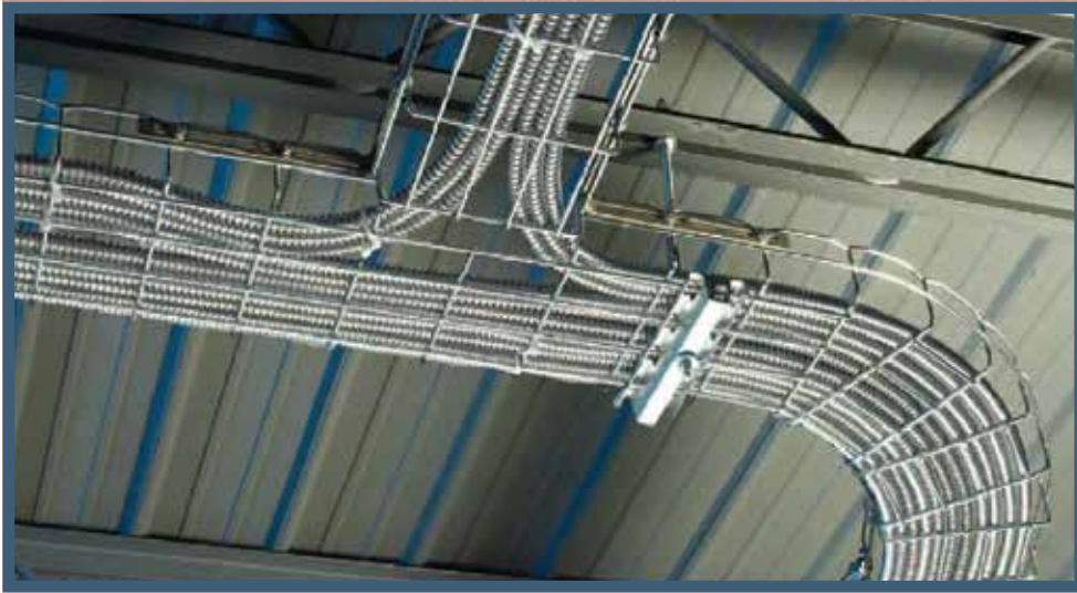
Wire Mesh Support System with Type MC cable
