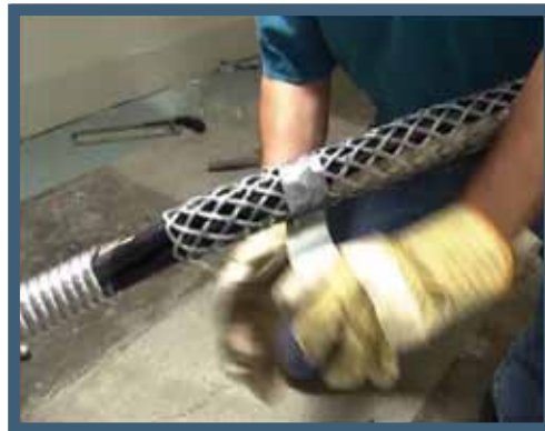
Securing basket grip to conductor assembly to avoid pulling conductors out of armor
