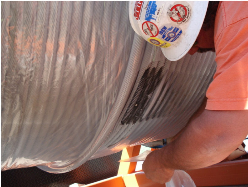
Figure 4. Water stain on conductor.
