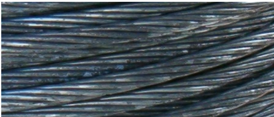
Figure 3. Oxidation on a conductor.
