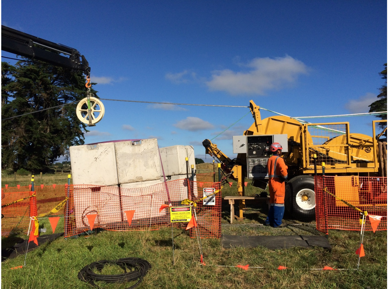
Figure 2: A full-size block should be used to avoid excessive bending around small guide rollers. Photo courtesy of Trans Power New Zealand.
