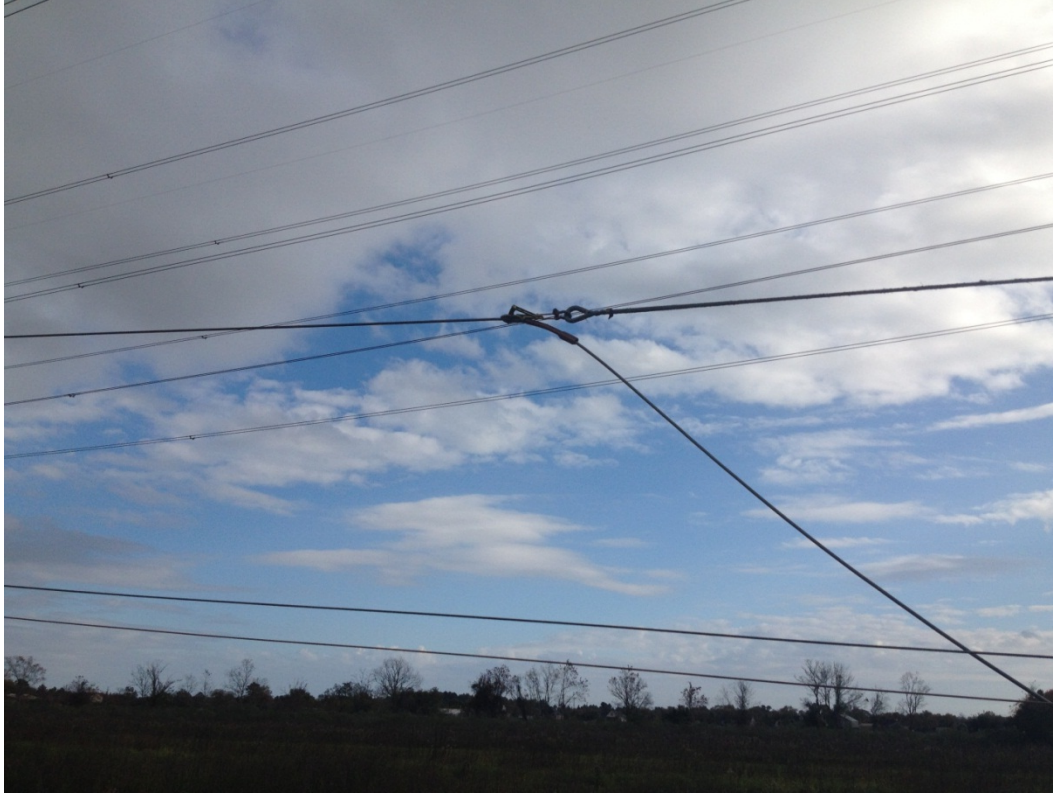
Figure 5: Care should be taken to ensure grips do not bend the conductor. Notice, the tail from the grip is trained at a gentle angle, and tension on the slack side is low to prevent excessive bending.
