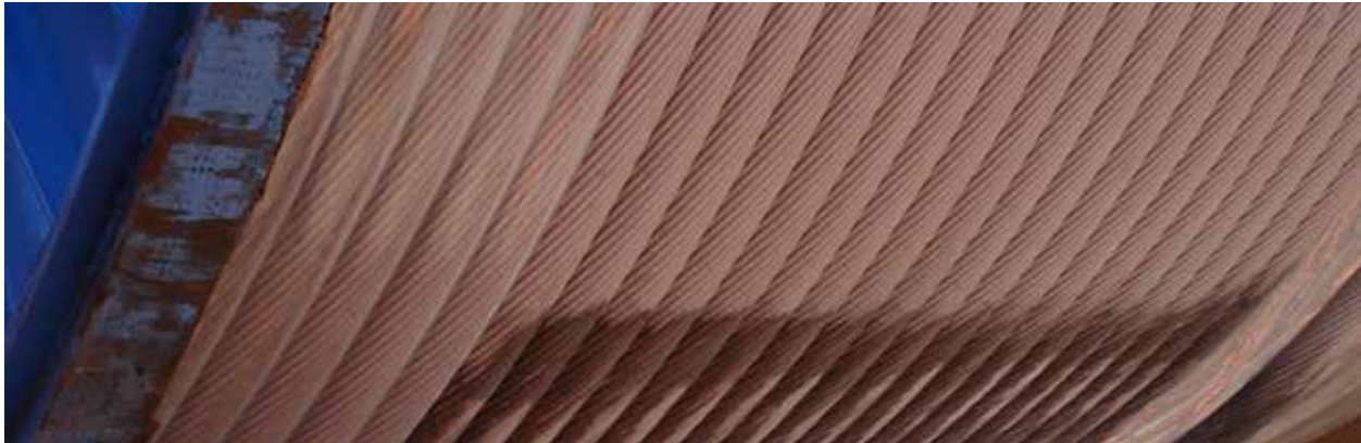
Figure 17. Water stain on conductor.
